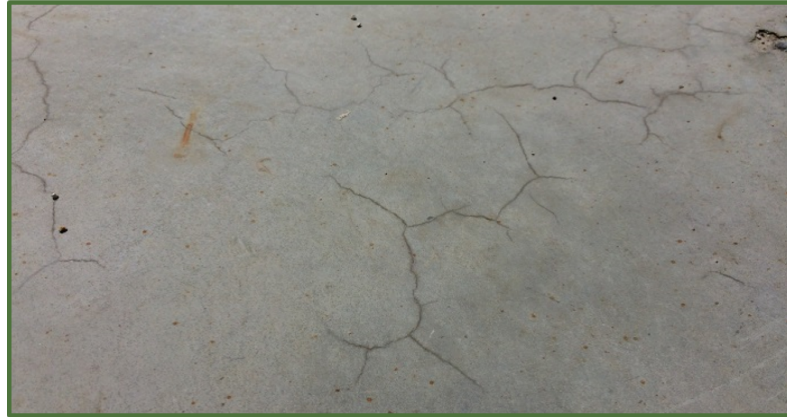
Figure 2.13: Thermal cracks in a thick slab
