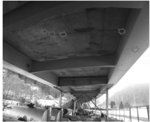
Figure 1. Monitoring system installed on Crêt de l'Anneau viaduct (Strain gauges are highlighted with clouds).
